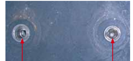
Drilled holes after 90 days salt spray test and after pull-out of the X-BT fasteners. These holes appear clean and no evidence of corrosion is visible.
